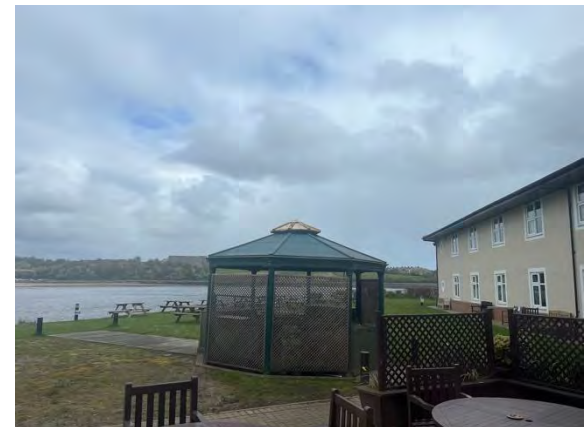
Existing Gazebo requires replacement
